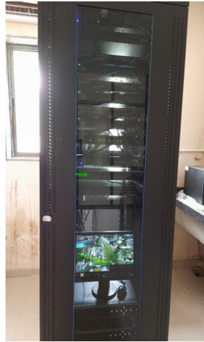
Server room rack with switches, Firewall
